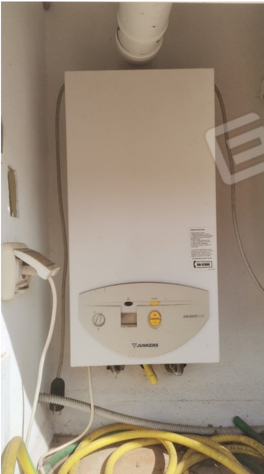
FIGURE 28: A9 CALDAIA GAS;
