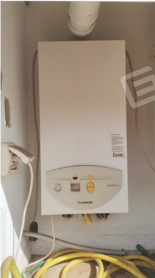
FIGURE 28: A9 CALDAIA GAS;
