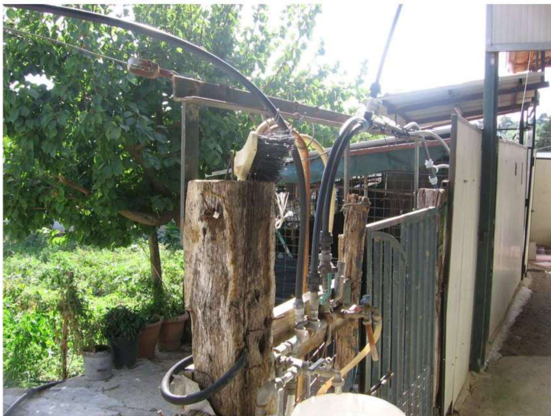
Strutture precarie abusive
