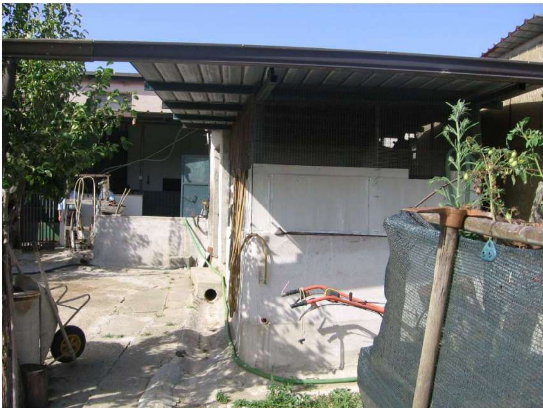
Strutture precarie abusive
