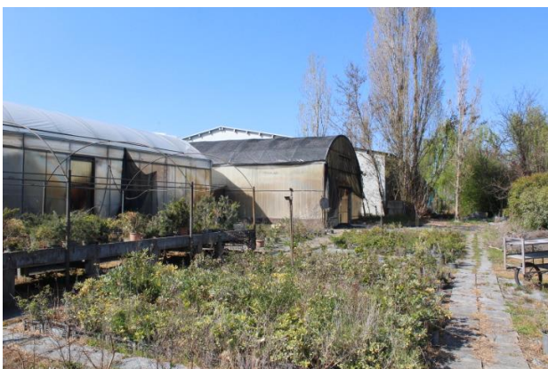
TERRENO LATO EST, SERRE ABUSIVE
