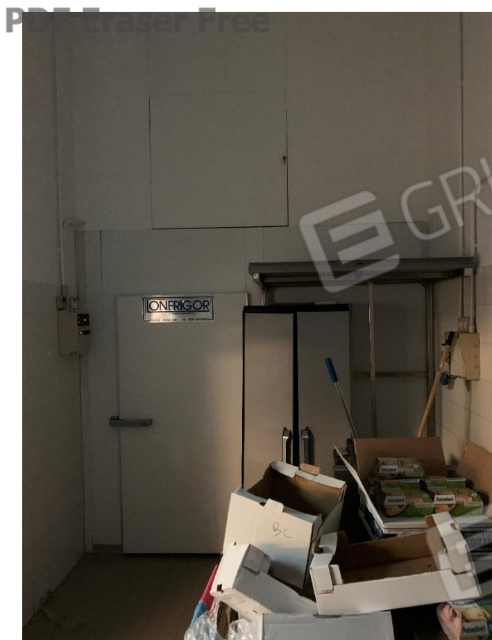
11 zona celle frigo piano terra
