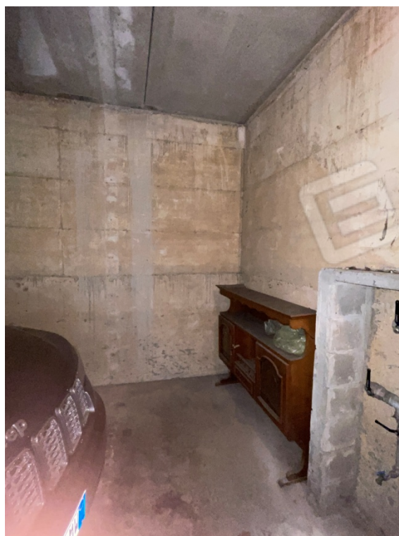
Sub.42 – locale caldaia
